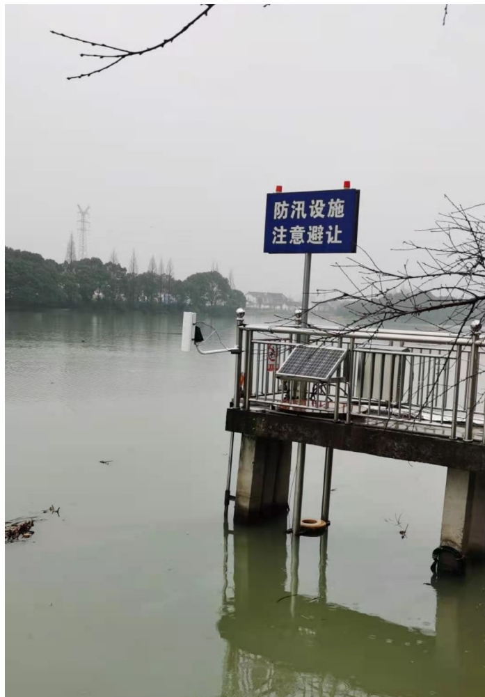
Figure 4 The test site of ATE7000 hyperspectral water quality monitor in Jiulong River, Zhangzhou, Fujian (without the liquid level monitoring module)
